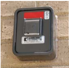
PICTURE OF A KNOX BOX AT A PROPERTY
